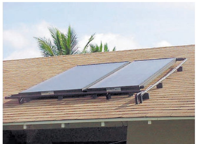
Two roof-mounted flat plate collectors.
